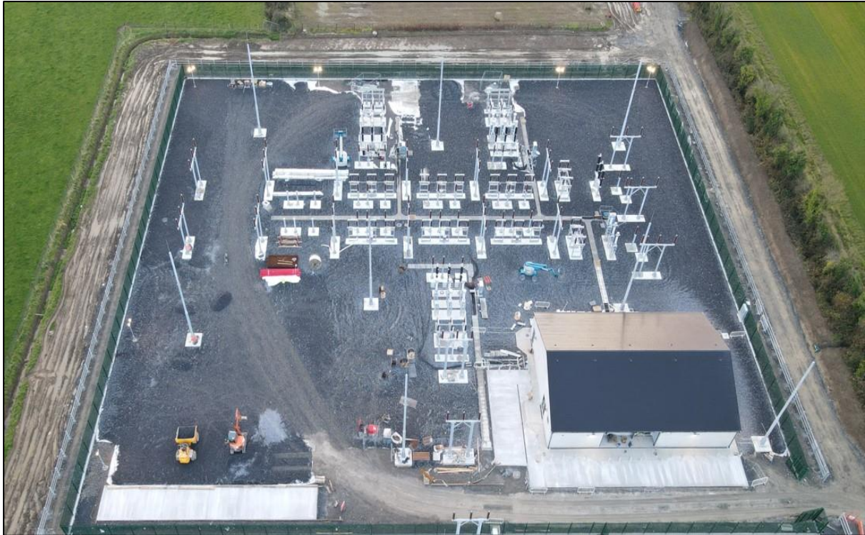
Figure 3.4: Example of a typical 110kV electricity Substation
