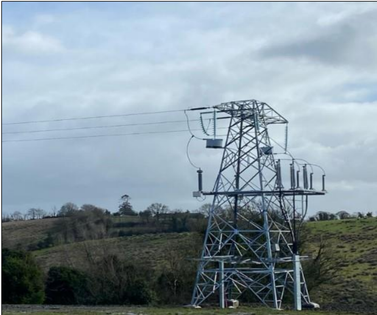
Figure 3.5: Typical Interface Mast
